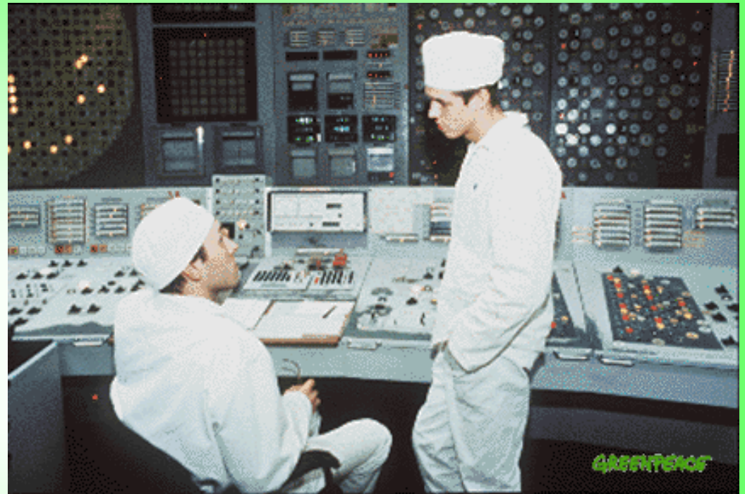
Inside the control room of 1st block. Chernobyl nuclear power station. Ukraine. 0.96.07.02.08 DEC 1995 CHERNOBYL UKRAINE D © Greenpeace/Shirley
