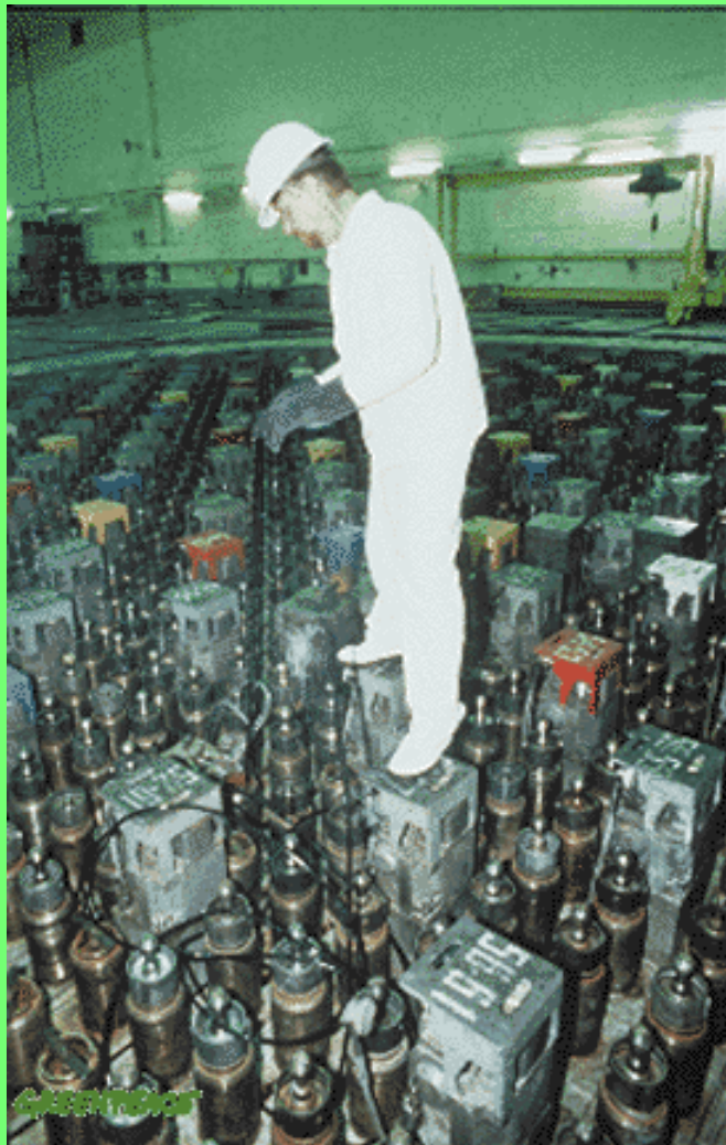
Inside 2nd reactor, checking graphite channels for cracks, Chernobyl, Ukraine. 0.96.07.02.10 DEC 1995 CHERNOBYL UKRAINE D © Greenpeace/Shirley
